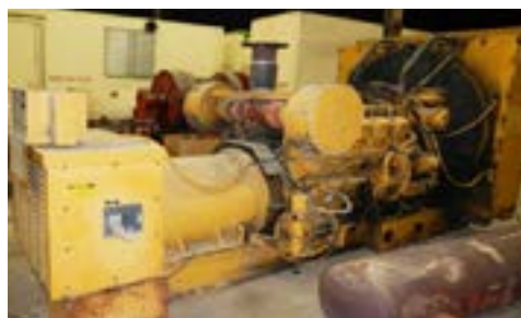
Caterpillar Genset Generator (Walton)
